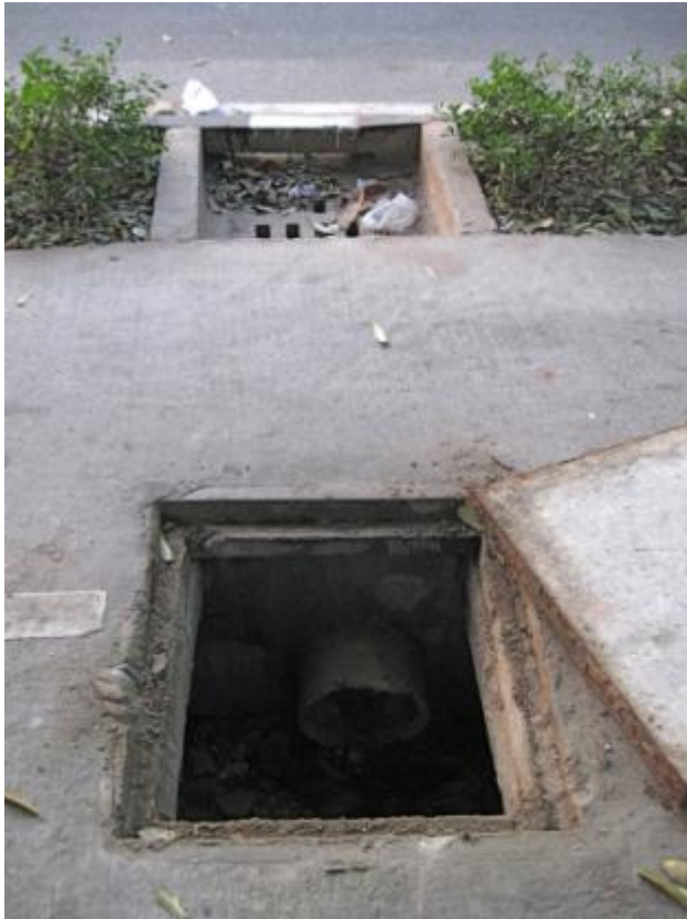
Figure 87: Storm water drain positioned below a cycle track, showing adjoining catch pit.
