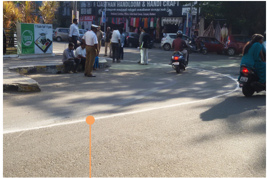
At intersections, kerblines marking should start 10m from the corner to allow for adjustment of the turning radius as required.
