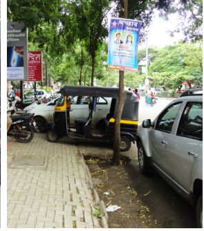
Dislocation of paver blocks due to poorly laid edge restraint i.e kerbs
