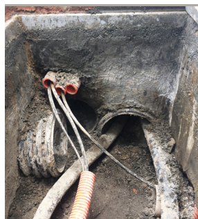
Multiple utility lines in one manhole due to lack of space
