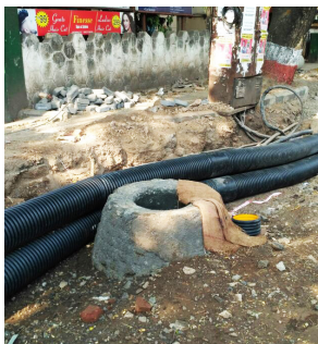
Conical manhole for stormwater
